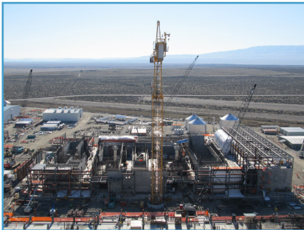
The High-Level Waste Vitrification Facility, shown here, is one of four major facilities under construction as part of the Hanford Tank Waste Treatment and Immobilization Plant, which is being built at the Hanford Site in Washington State. The plant will treat radioactive and hazardous waste currently stored in 177 underground tanks.
