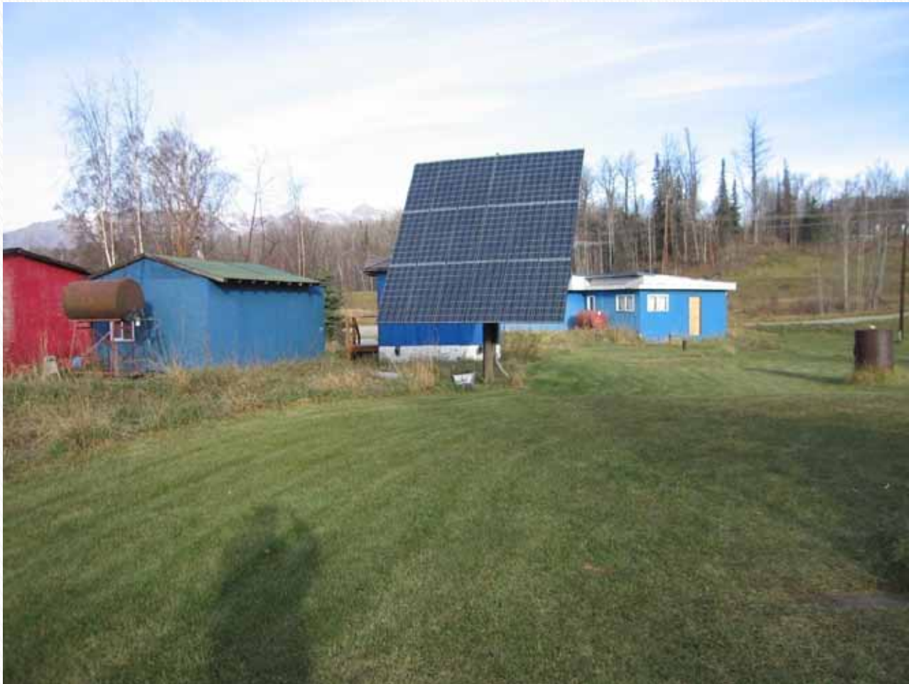
Another view of the Solar Tracking System
