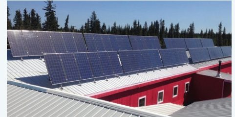
In addition to energy efficiency upgrades on the Tribal Hall building, GZGTG worked with Tanana Chiefs Conference to install solar panels that, during the sunny months of the year, are expected to produce more power than the building uses each month, offsetting an estimated 1,300 gallons of diesel-generated power annually. Photo from Dave Pelunis-Messier, Tanana Chiefs Conference
