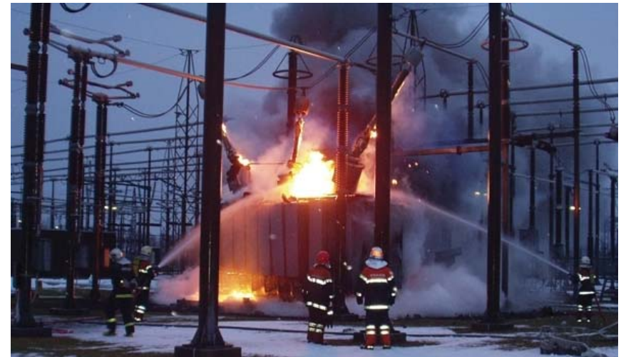
Large Power Transformer Fire from Bushing Failure
