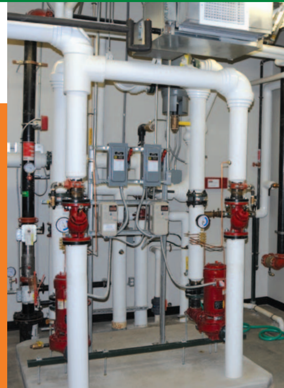
The geothermal heat pump system provides heating and cooling to the building.
