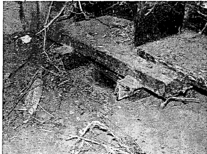
Figure 28. Movement at the bridge bearing (Photo: Chadwell).
