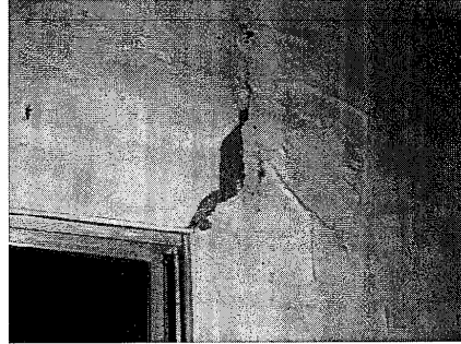
Figure 10. Typical cracks in the stucco finish (Photo: Chadwell).
