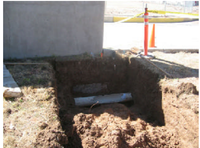
Excavation Event Involving a Water Pipe
