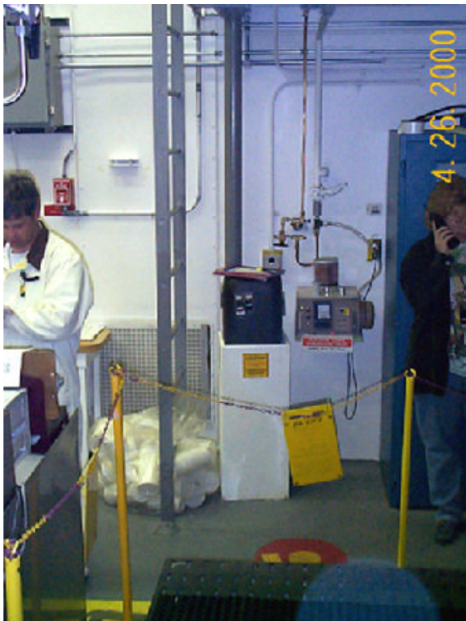
Continuous Air Monitors
