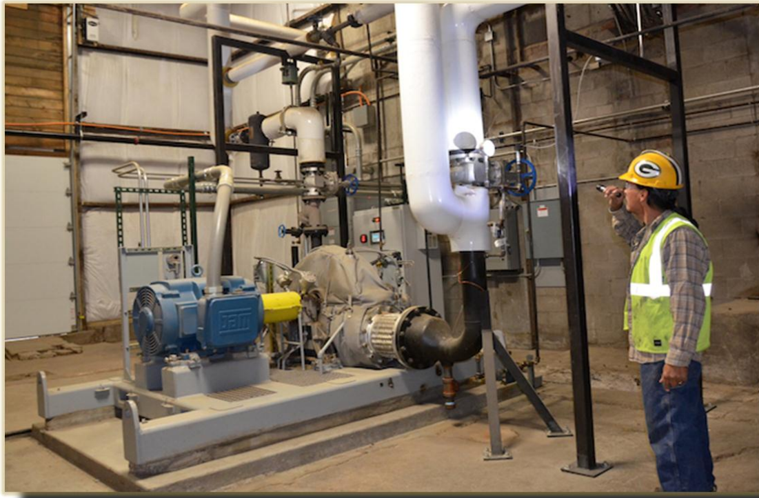
Figure 9 – Backpressure Steam Turbine Generator
