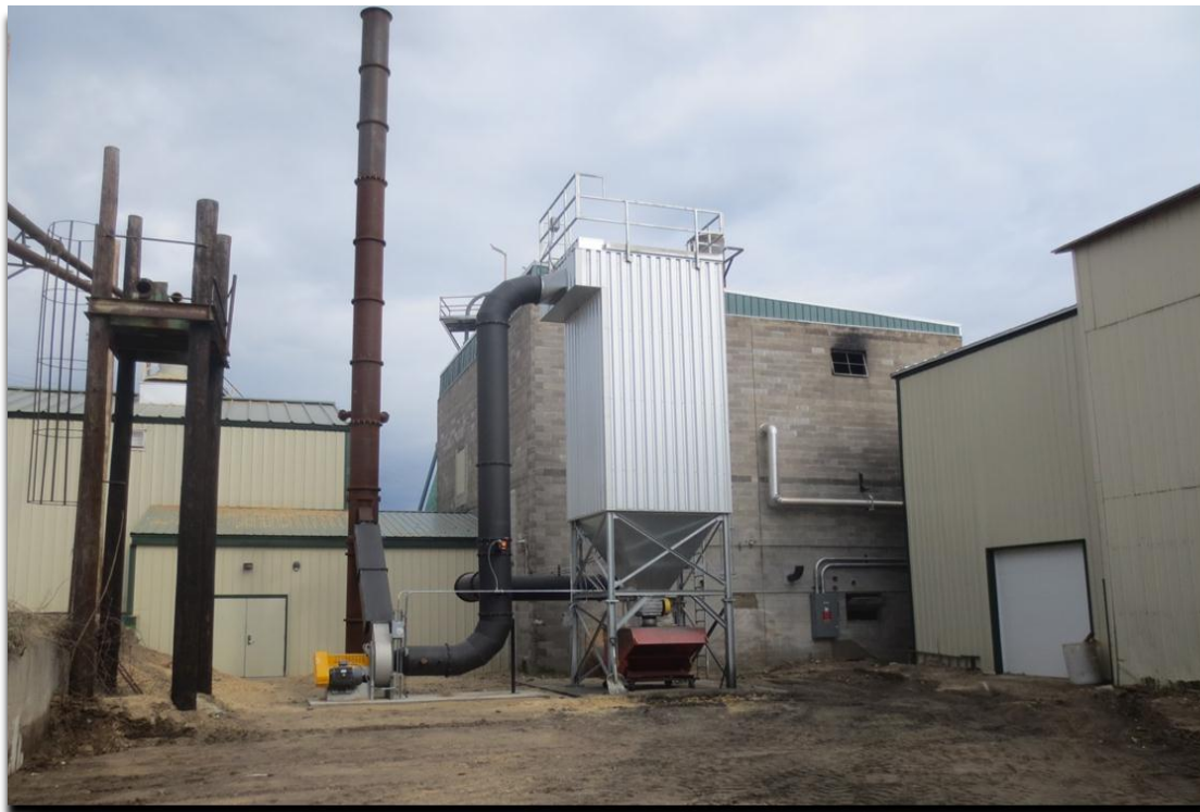
Figure 10 – Bag House and New Stack
