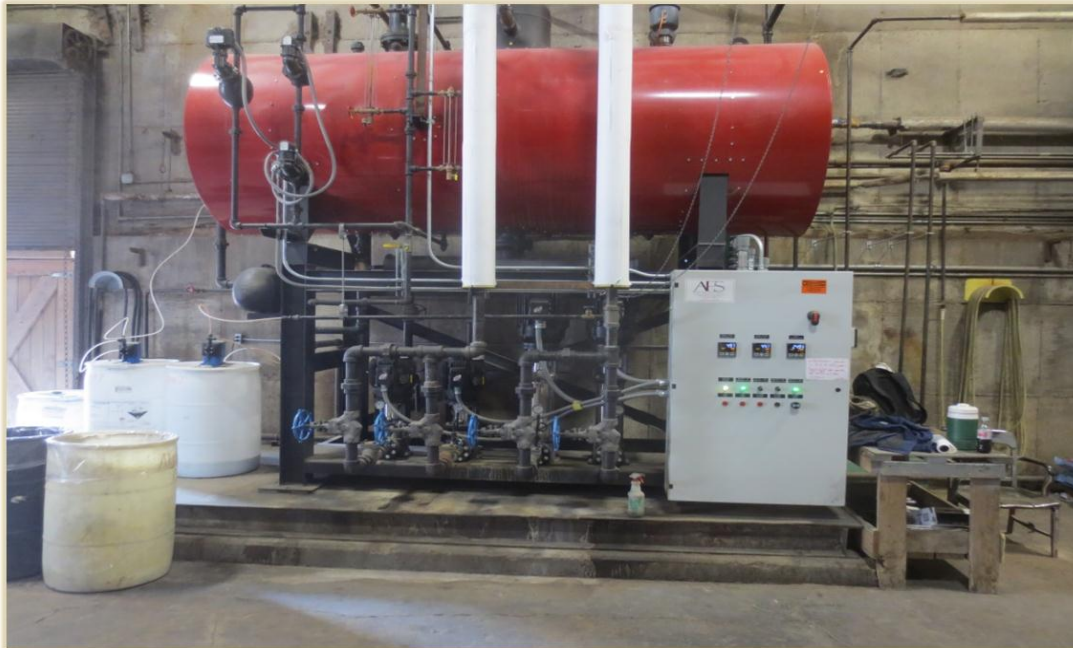
Figure 8 – Deaerator Serves New and Existing Boilers
