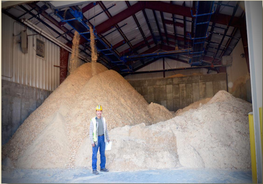
Figure 7 – New Fuel Storage
