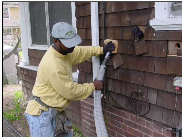
The one-hole method using a tube long enough to reach to the furthest corner of the cavity is the best way to dense pack walls
