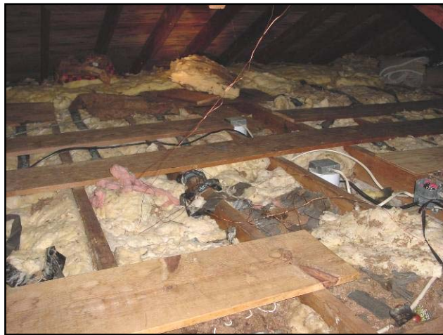
Some attics require much preparation work before they can be blown with cellulose
