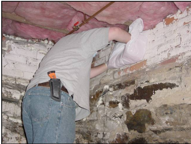
Stuffing the band joist area with an “insulation pillow” (a plastic bag filled with fiberglass)
