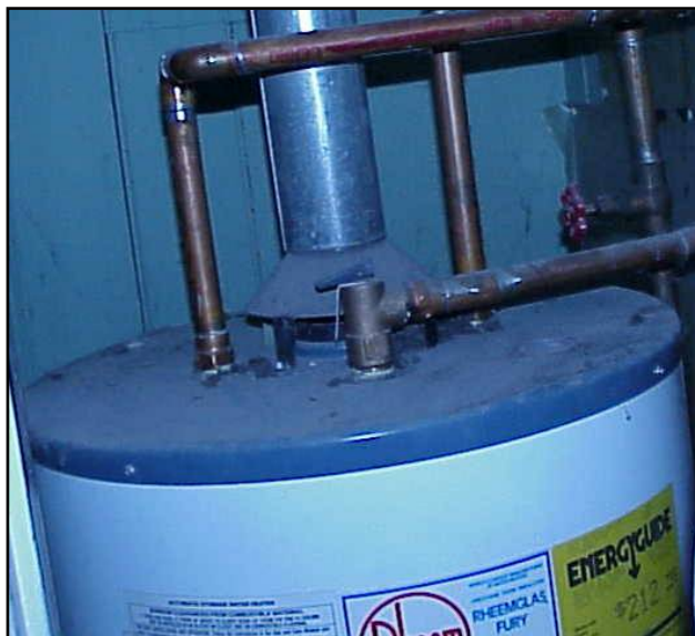
Stand-alone gas water heaters are the most likely appliance to suffer draft reversal
