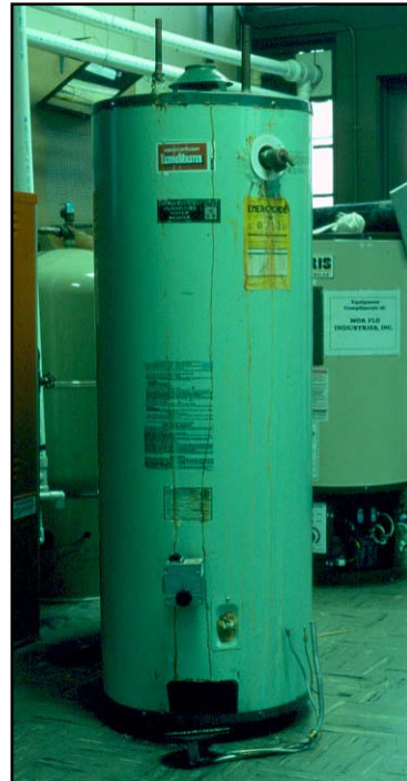
Old and leaking water heaters should be replaced
