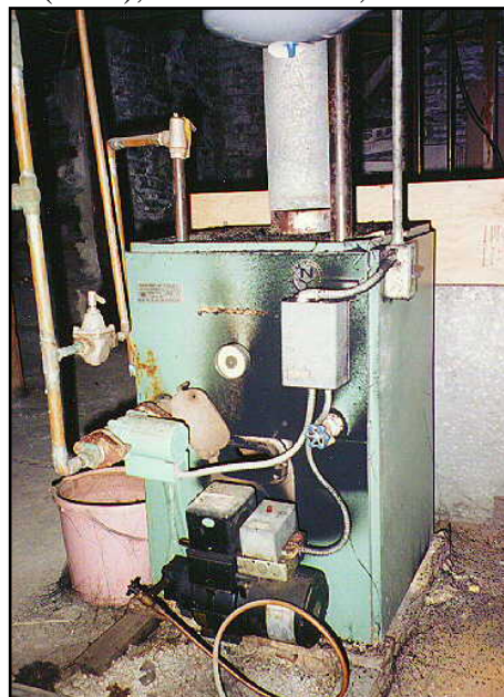
Obvious evidence of drafting failure
