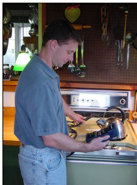
Testing gas oven for CO emission level
