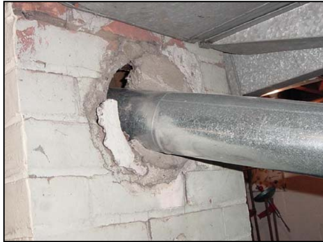
An example of a very hazardous venting problem
