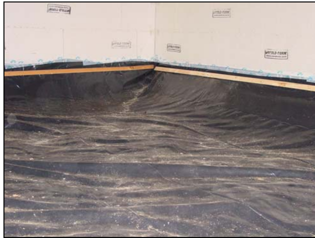
Ground cover sealed to foundation walls
