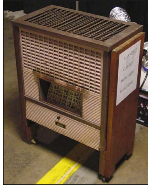
Replace old and hazardous space heaters with direct-vent, sealed combustion units
