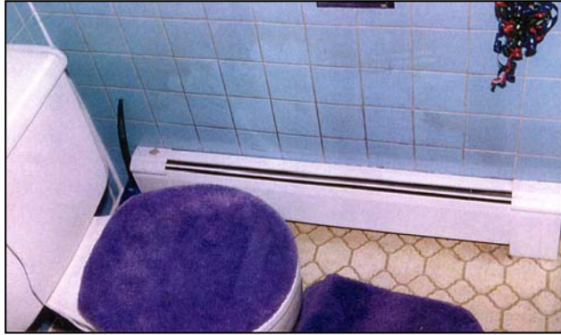
Hot water baseboard distribution usually operates with a maximum water temperature from 180 to 200°F
