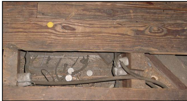
Even if there is attic flooring, knob-and-tube wiring and attic bypasses must be found and treated before insulation is added
