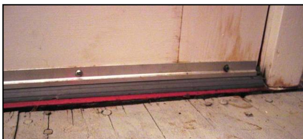
Exterior door threshold sweep
