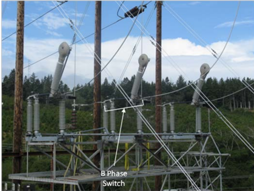
Figure 5: Structure 46/5S Switch B447
