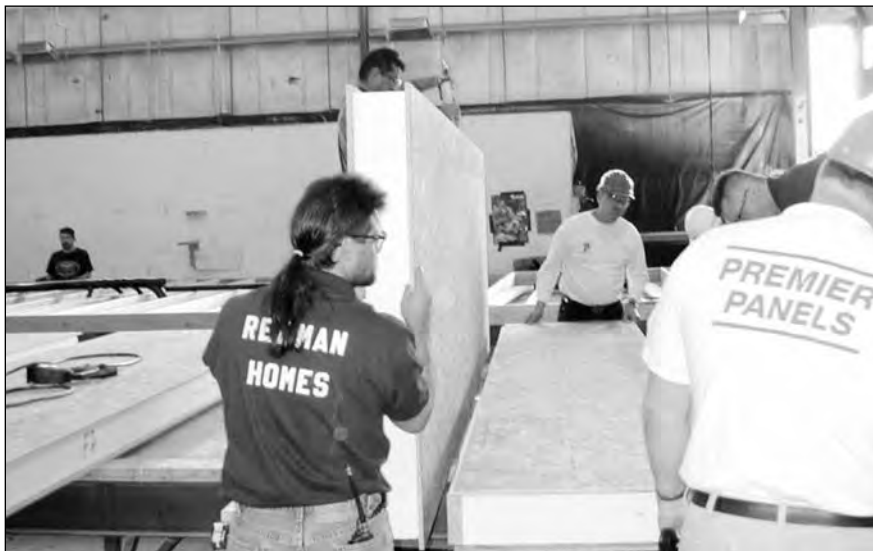
The Redman factory's first workstation is for floor layout. This photo shows the roughly 4 foot by 14 foot floor panels being assembled with 2 x 6 splines between the panels.
