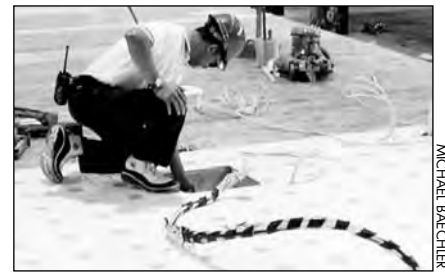
Work continued on interior components such as flooring, interior walls, plumbing, and electrical while the exterior walls and roof were being prepared.
