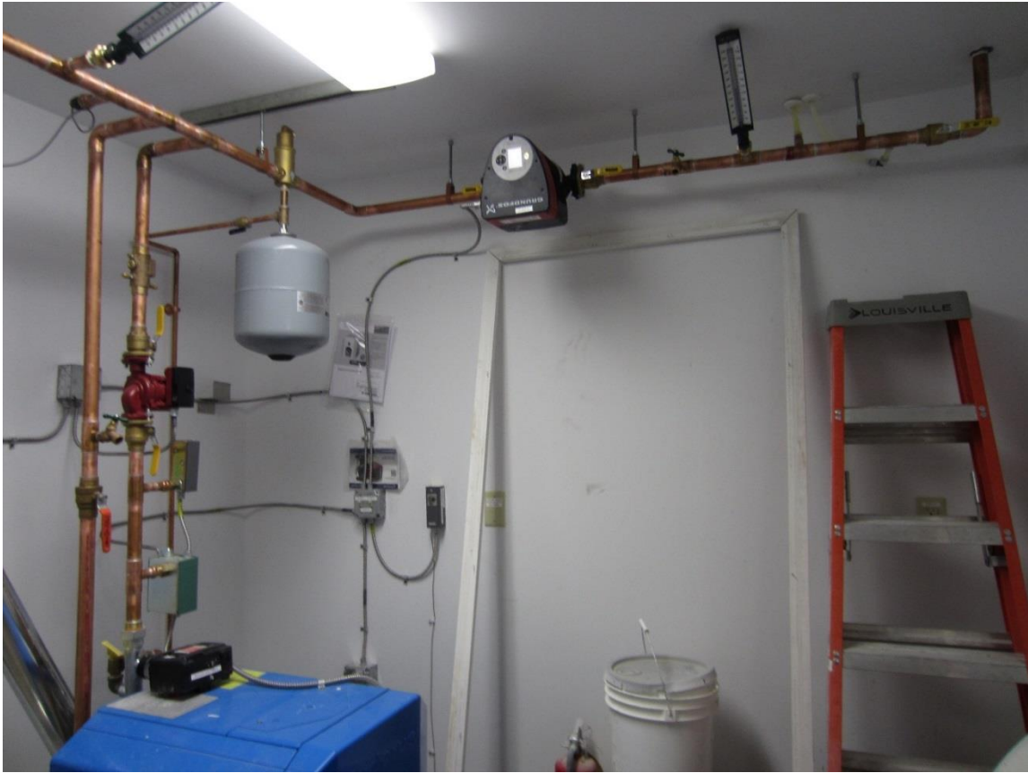
Figure 14 The buildings new heating system (downstairs).
