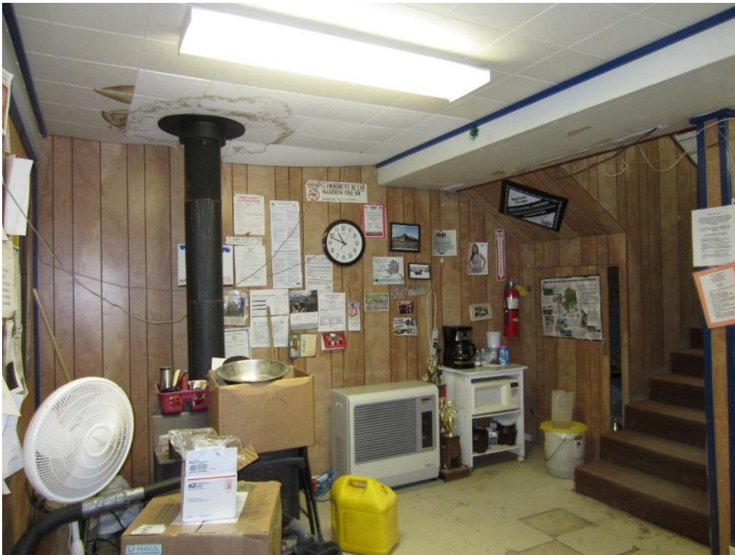
Figure 6 Koyukuk Office downstairs with woodstove, and monitor. Note water damage from roof leak around stove pipe vent.
