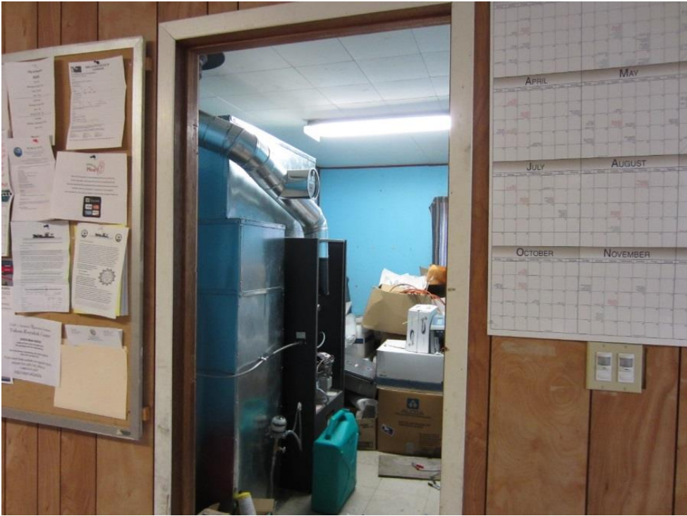
Figure 7 Koyukuk old furnace located upstairs
