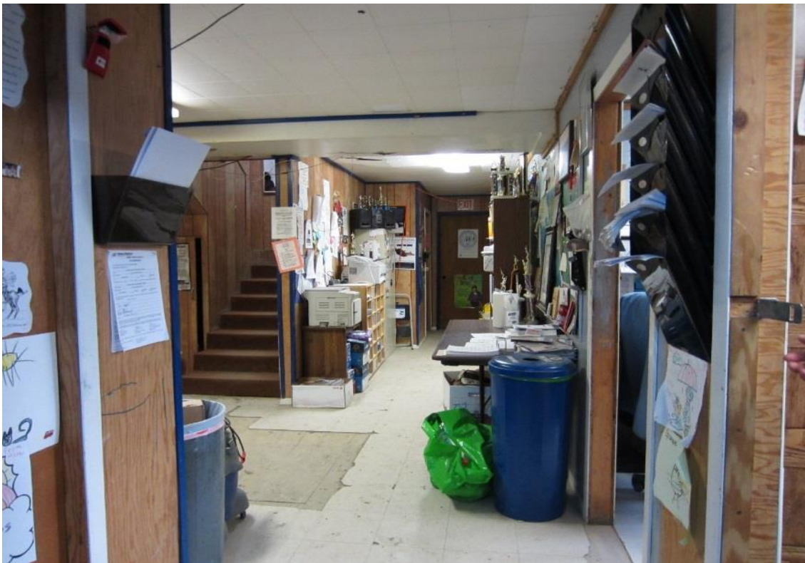
Figure 4 Koyukuk Office 1st floor prior to renovation note damaged floor.
