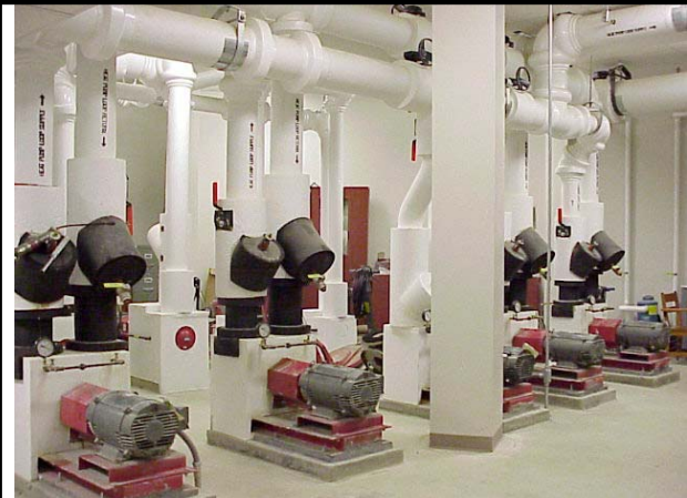
Hookup and Commissioning – Integration with Indoor System
