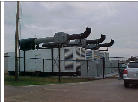
Three 2 MW Diesel Generator Sets (serve as start-up units for the two 12.5 MW gas fired steam units.)
