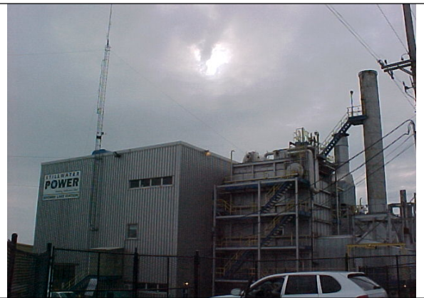
Two 12.5 MW Gas Fired Steam Generator Units
