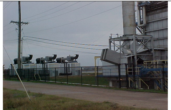
Stillwater Power Generation Units
