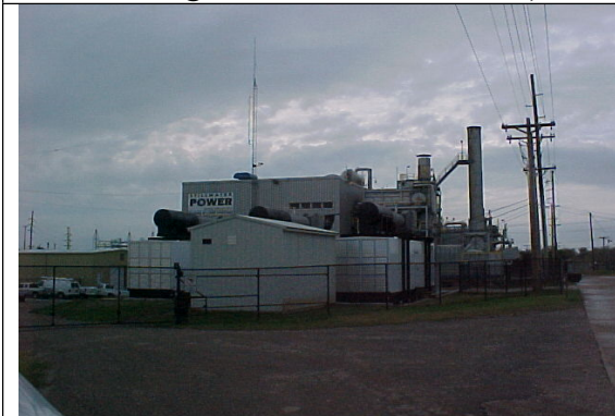
Stillwater Power Generation Units
