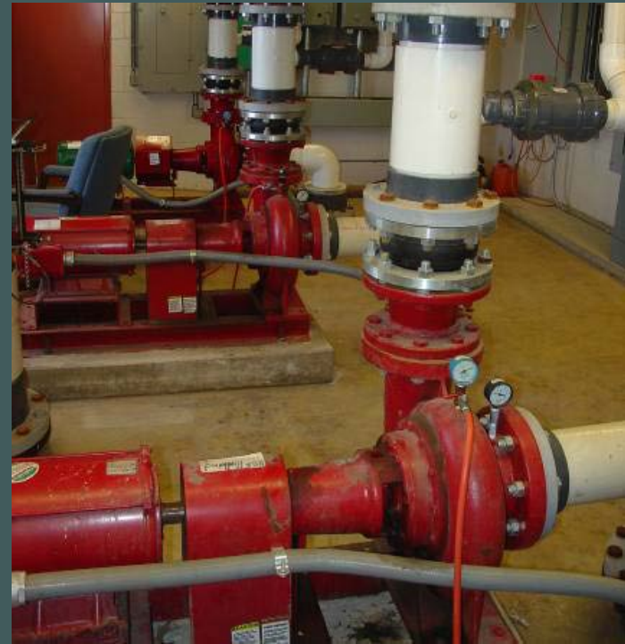
3 x 15 HP Lake Pump in New Hatchery
