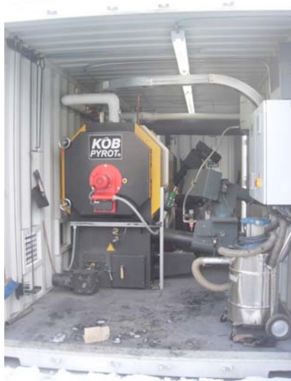
figure 2.7, a Köb boiler installed in OR
