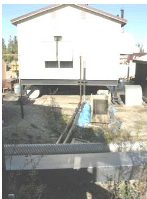
figure 2.8, a piping utilidor
