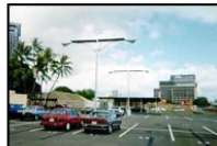
Solar lighting in the PJKK federal building parking lot
