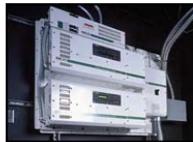
A Typical Inverter
