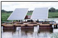
A solar-powered water pumping station for irrigation
