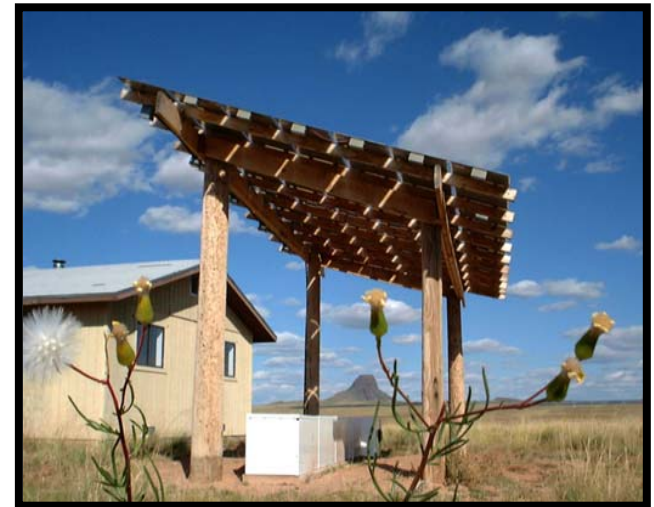
Solar Installation on Navajo Nation
