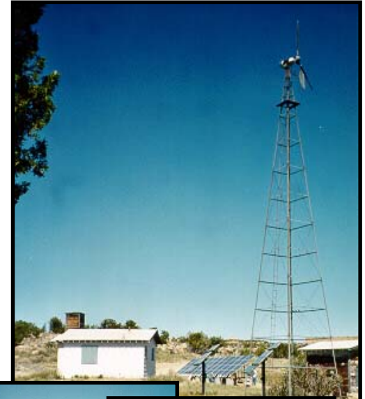
Pueblo of Laguna (Majors Ranch) Solar and Wind Installations
