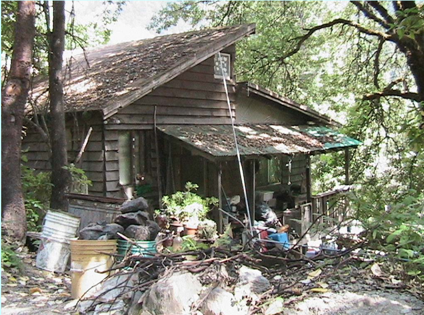
New Village Weitchpec housing unit that will probably not meet UBC.
