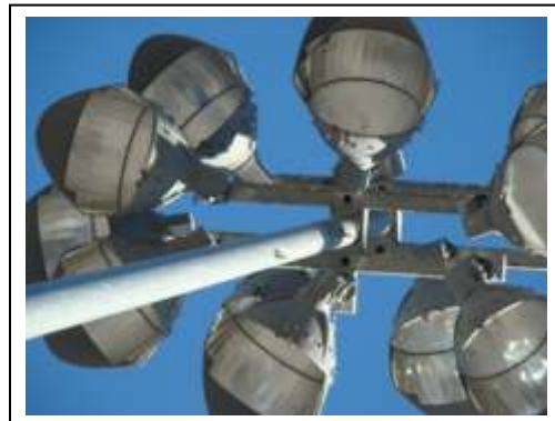
Sports field lighting
