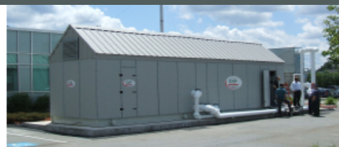
■ A CHP TR250 trigeneration unit.
