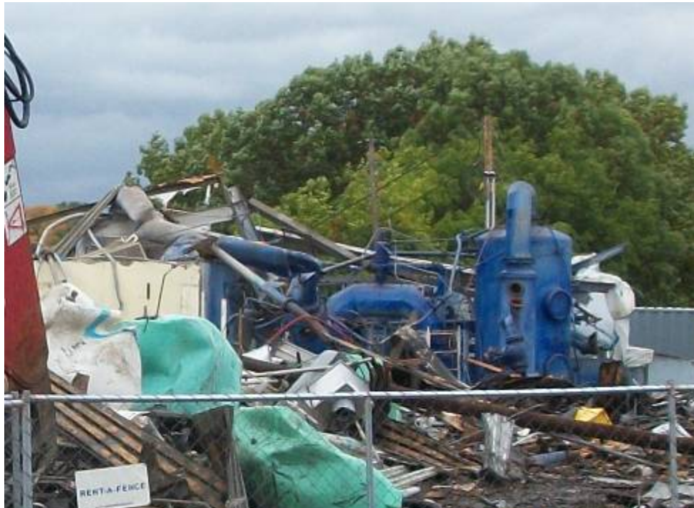
Figure 3-1: Incomplete Application of Fixative to Separator Columns September 29, 2010
