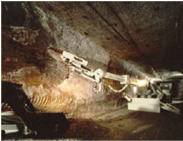
Scaler Miner Removing Loose Rock in the Waste Isolation Pilot Plant Underground
