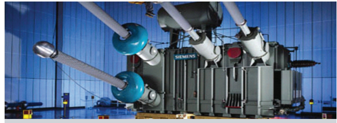
Figure 2. High-voltage direct converter (HVDC) (Courtesy: Siemens AG)
