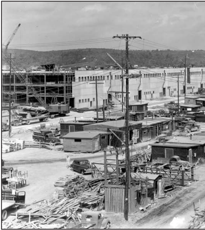
K-25 Gaseous Diffusion Plant Under Construction at Clinton. Reprinted from Richard G. Hewlett and Oscar E. Anderson, Jr., The New World, 1939-1946 , Volume I of A History of the United States Atomic Energy Commission (University Park: Pennsylvania State University Press, 1962).
