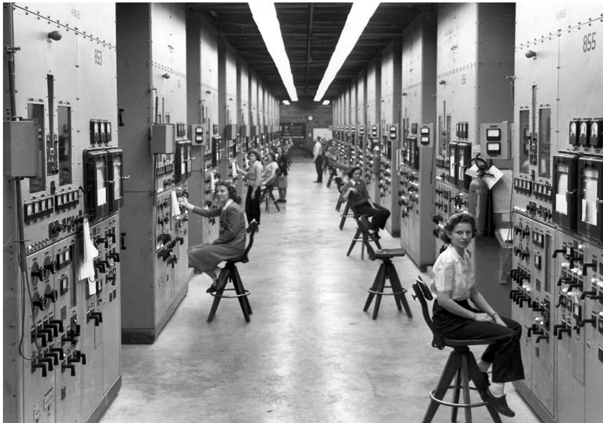
Y-12 control room
