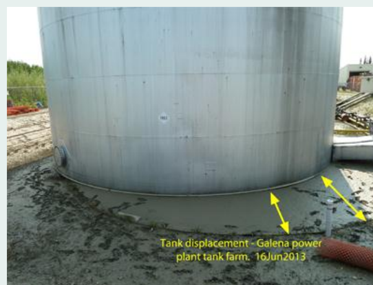
Figure 2-10. Galena power plant fuel storage tank shifted by ice jam flooding in 2013.
