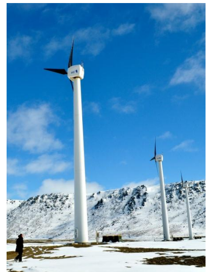
Figure 2-7. AVEC installed wind turbines in Gambell in 2009 to supplement diesel generation. Source: NPS 2013
