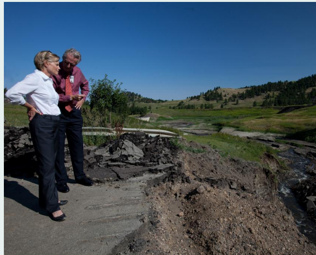
Figure 5-5. Heavy rainfall washed out roads on Rocky Boy’s Reservation in June 2010. Source: FEMA 2010
