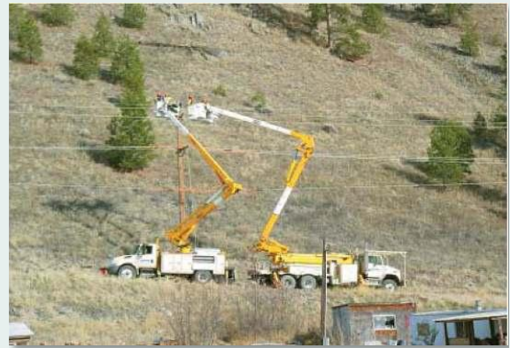
Figure 5-2. Employees of Mission Valley Power perform maintenance on power lines in the service area.
