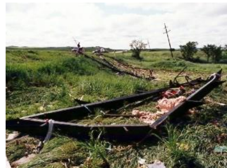
Figure 5-3. A tornado snapped utility poles when it hit the Pine Ridge Reservation in South Dakota in 1999. Source: NOAA 2010
