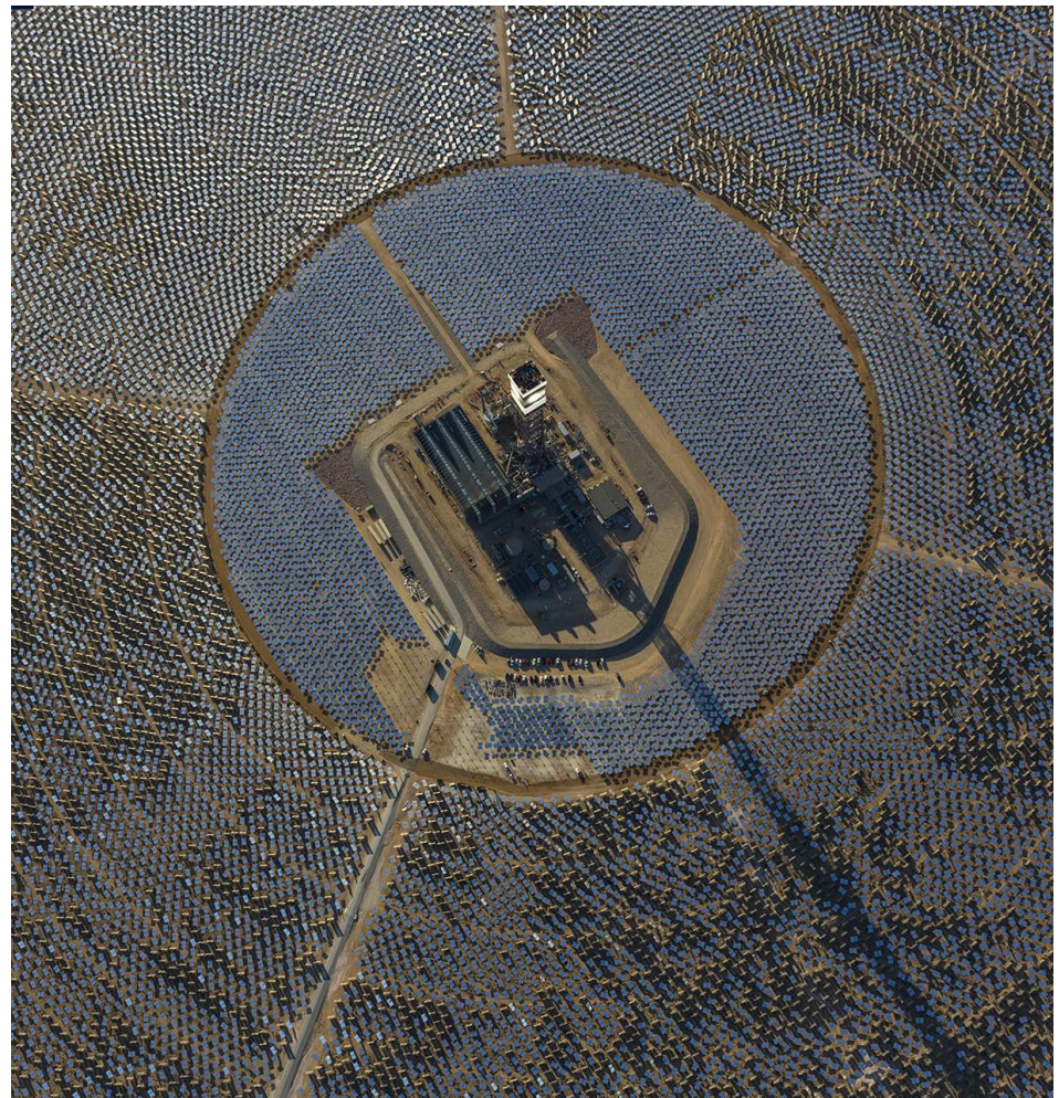
Aerial view of one of the Ivanpah power towers in Ivanpah Dry Lake, California. Photo Credit: BrightSource Energy
