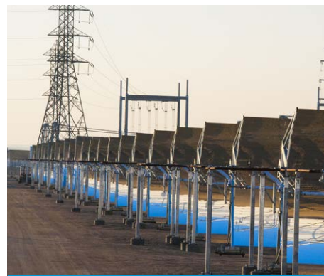
Mojave, Photo Credit: Abengoa Solar, Inc.
