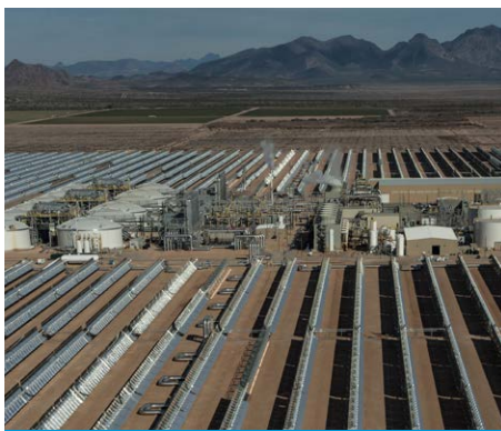
Solana, Photo Credit: Abengoa Solar, Inc.
