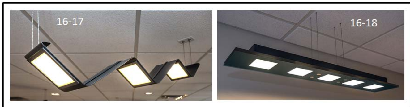
Figure 2. Photos of the two supplementary OLED luminaire types tested. Photos courtesy OLEDWorks Inc. and DeJoy, Knauf, & Blood, LLP.
