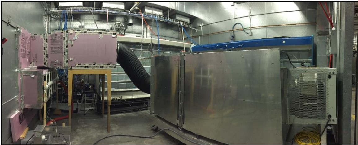
Figure C.2. As installed R-410A unit.
